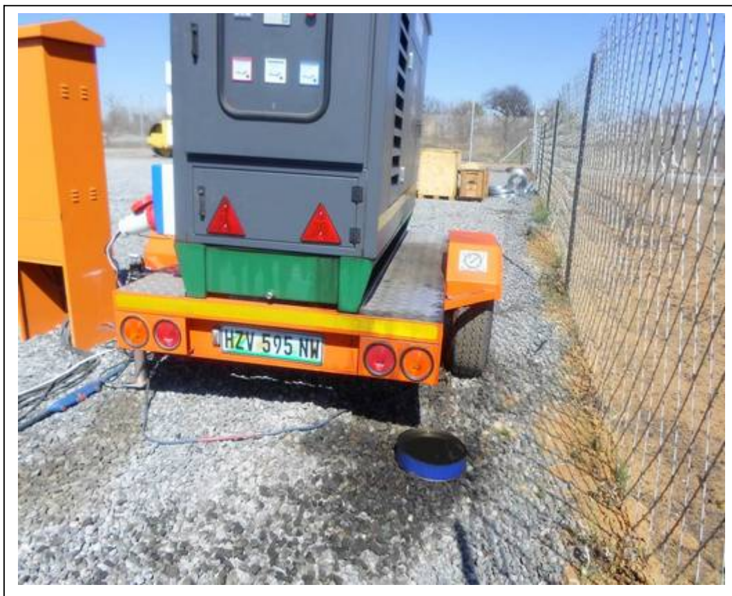
Figure 1: Oil spillages surrounding the generator
