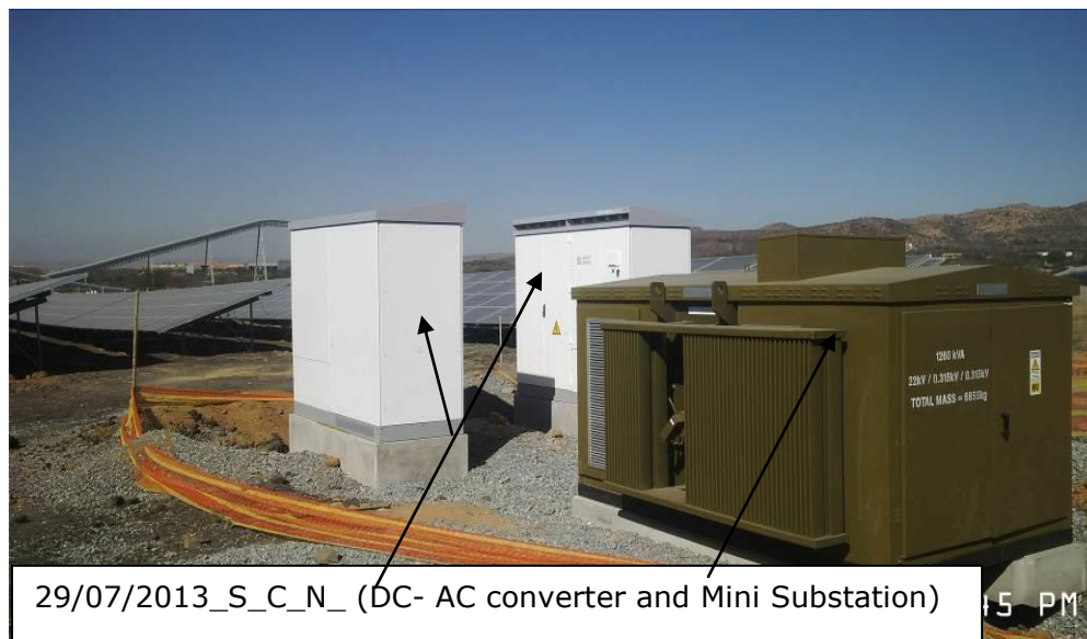
Figure 1: DC- AC Converter and Mini Substation
